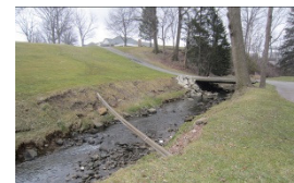
Degraded Euclid Creek tributary running through Acacia - a great opportunity for restoration
