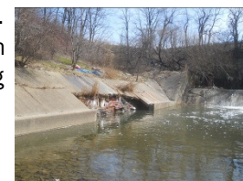
Repair of concrete at the Euclid Creek E. 185th Street Spillway is one of NEORS D's 'first out' emergency repair projects in 2013
