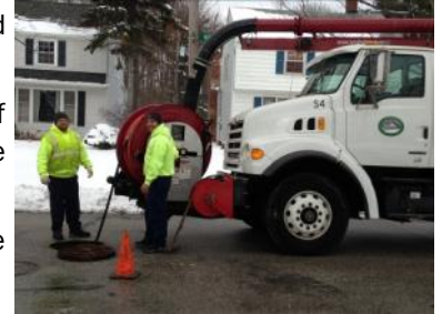
Rob Trybus and Matt Gerome, Lyndhurst Service Department Staff, working hard to protect infrastructure and Euclid Creek
