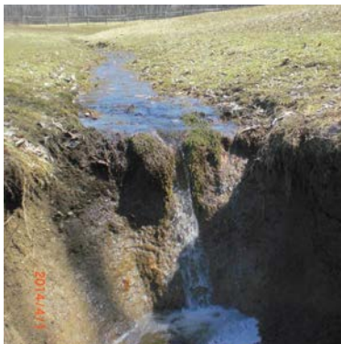
Downcutting occurring before restoration
